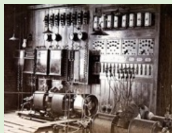
Dentokyo transmission panel
