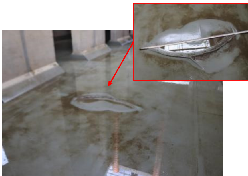
Waterproof coating bubbles
