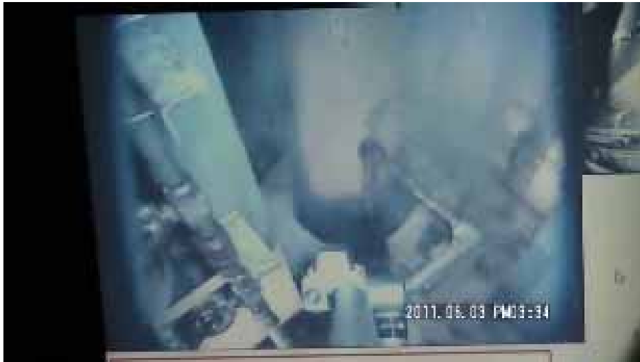
Steam release from the penetration on 1 st floor (photo as at Jun. 3, 2011)
