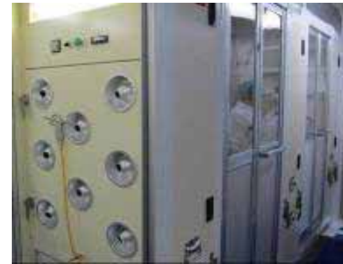
Air shower in rest place
