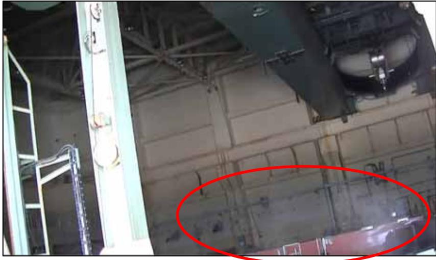
Steam release from right above the reactor on 5 th floor (photo as of Sep. 17, 2011)
