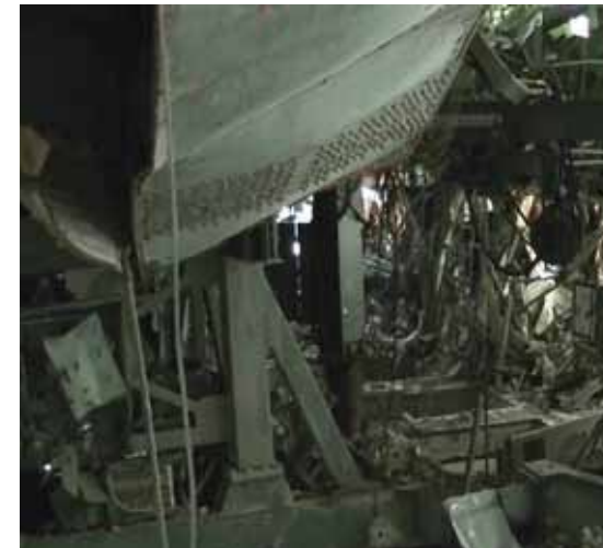
Photo taken in October 2012 (during the investigation of the operation floor utilizing a balloon)
