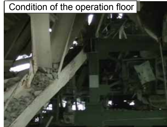
Photo taken in October 2012 (during the investigation of the operation floor utilizing a balloon)
