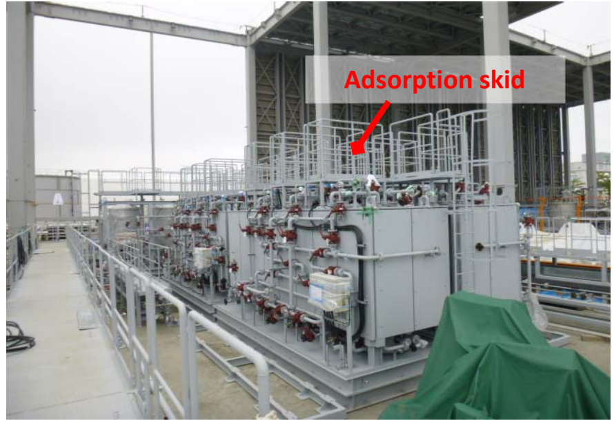
Adsorption tower of improved ALPS building (photo taken on Aug 15 2014)
