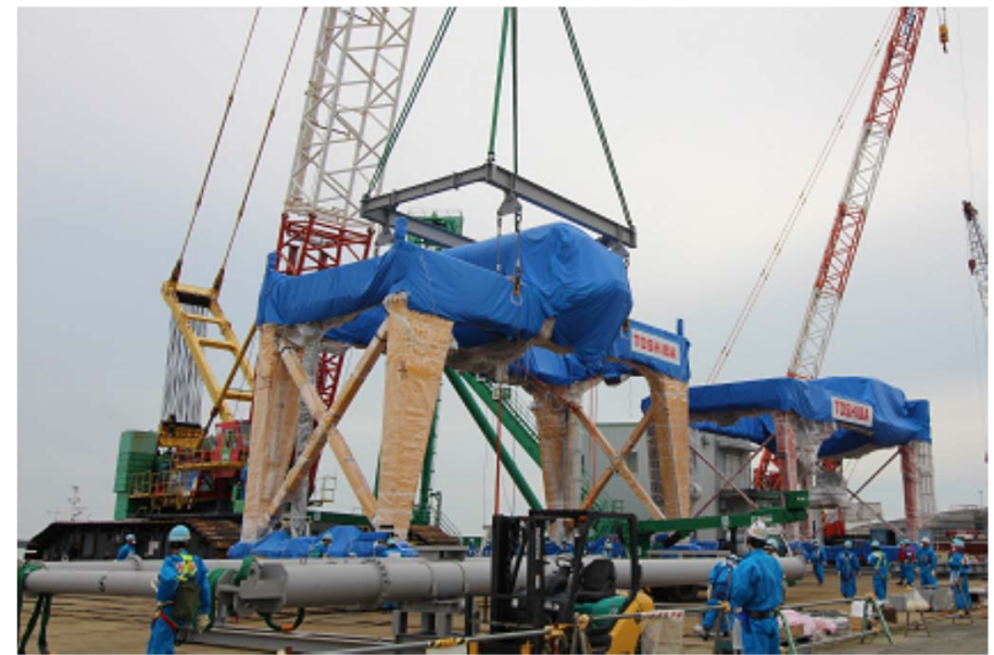
The crane (left) and fuel handling machine (far right)
