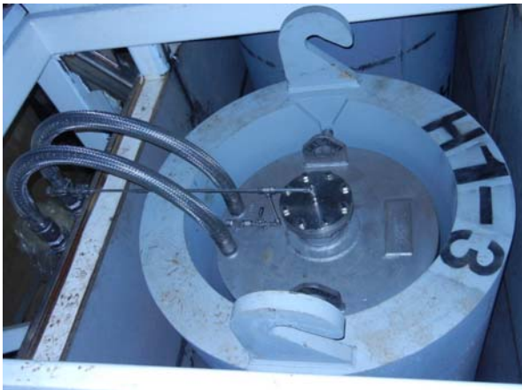
H skid (Cesium adsorption tower) June 6, 2011 Photo by TEPCO
