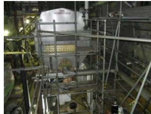
Disk filter (Decontamination instruments) June 5, 2011 Photo by TEPCO
