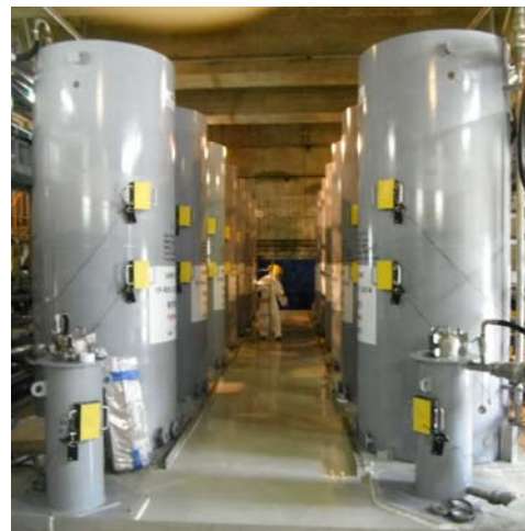
Cesium adsorption towers and media filter August 2, 2011 Photo by partner company
