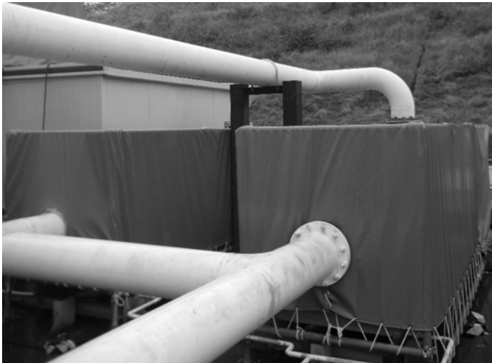
Exhaust ventilation apparatus, decontamination facility
