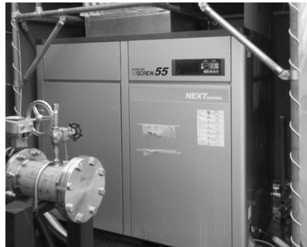
Compressor, decontamination facility
