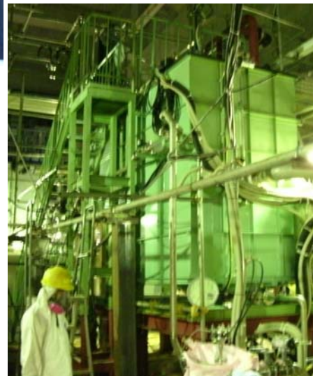
Super high speed coagulation settling decontamination facility (Decontamination instrument) June 15, 2011 Photo by TEPCO
