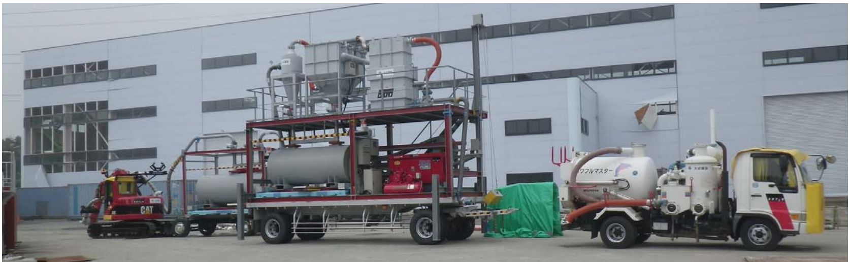
<Full view of dust collector system>
