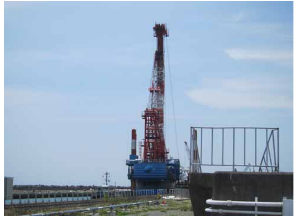
Impermeable wall piling ship Photo taken by a TEPCO employee on June 18, 2012
