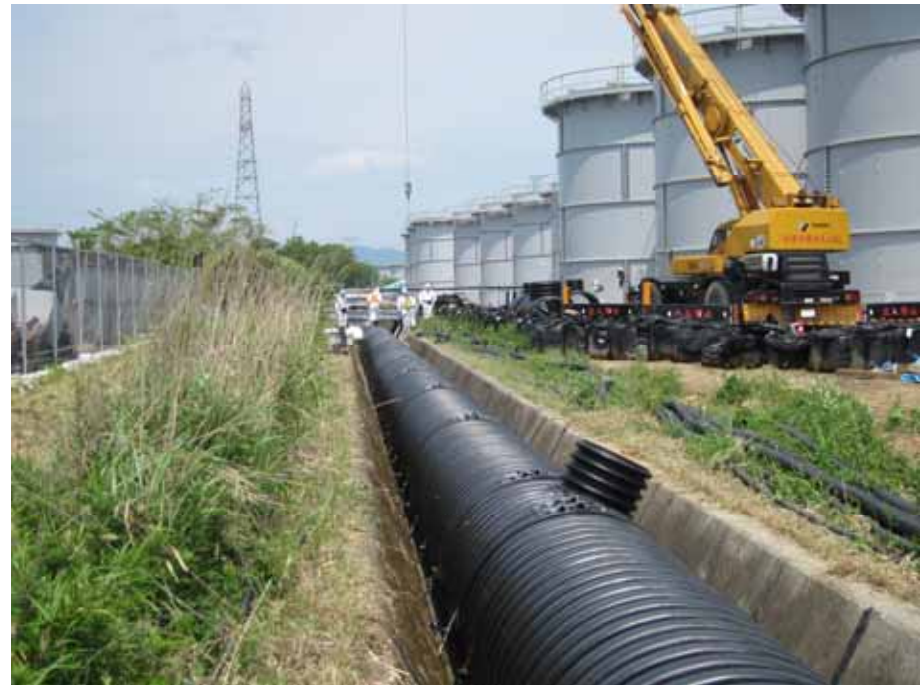
-2 PE pipe installation condition Photo taken by a TEPCO employee on June 18, 2012
