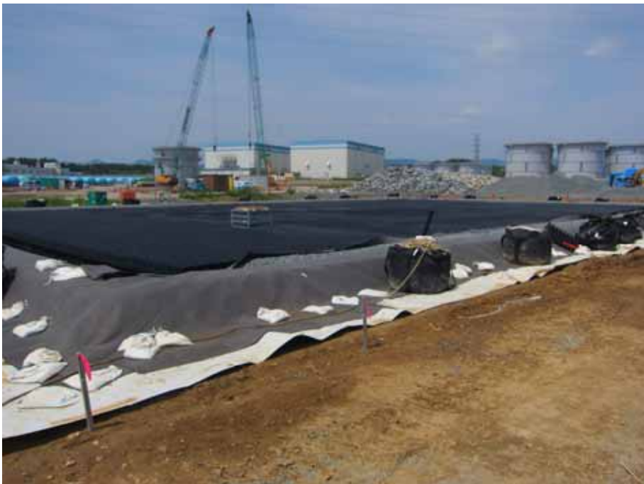
-1 Underground water storage tank installation Photo taken by a TEPCO employee on June 18, 2012
