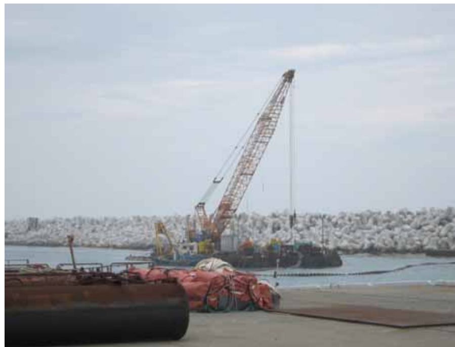
-2 Marine soil covering work: Solidified soil placing ship Photo taken by a TEPCO employee on June 7, 2012
