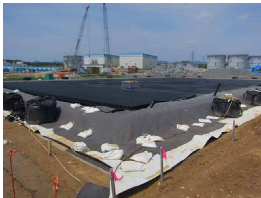
-2 Underground water storage tank installation Photo taken by a TEPCO employee on June 18, 2012
