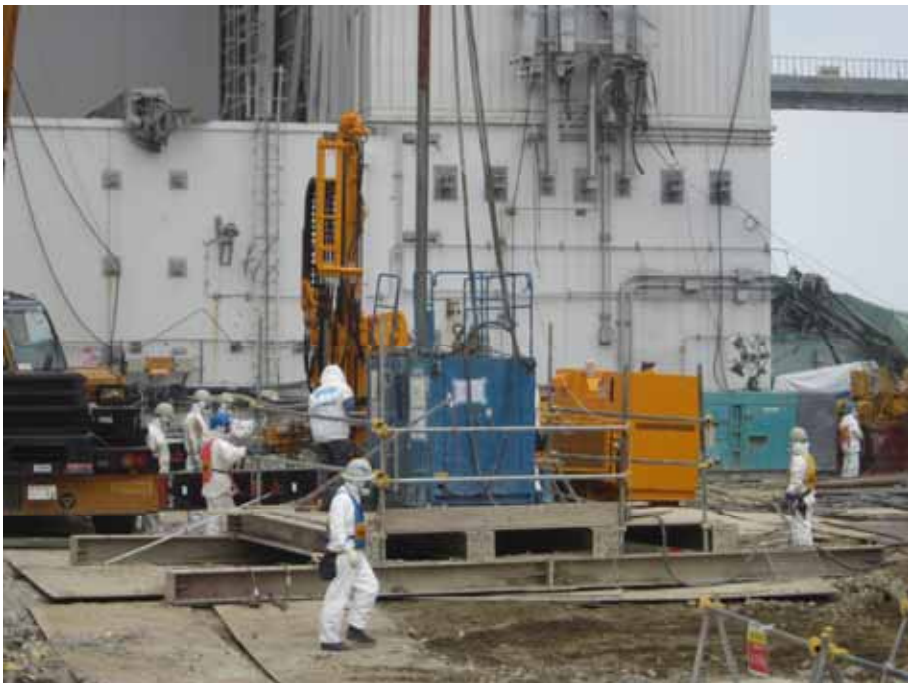
-1 Unit 4 south side foundation improvement work: Foundation improvement equipment Photo taken by a TEPCO employee on June 7, 2012
