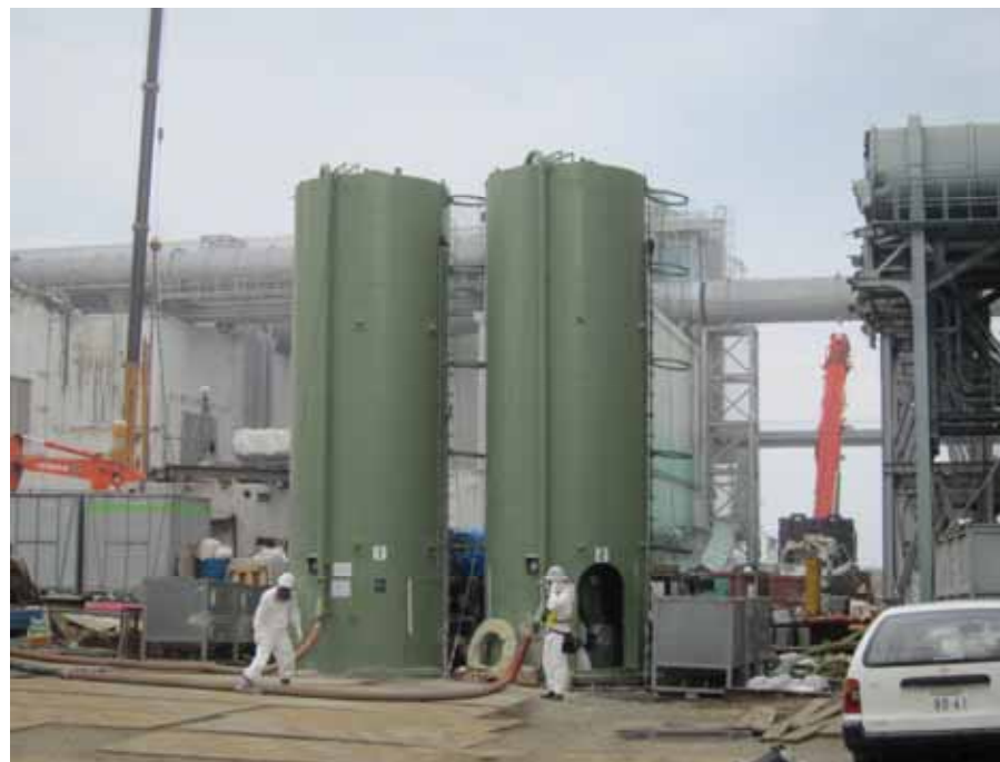
-2 Unit 4 south side foundation improvement work: Cement silo Photo taken by a TEPCO employee on June 7, 2012
