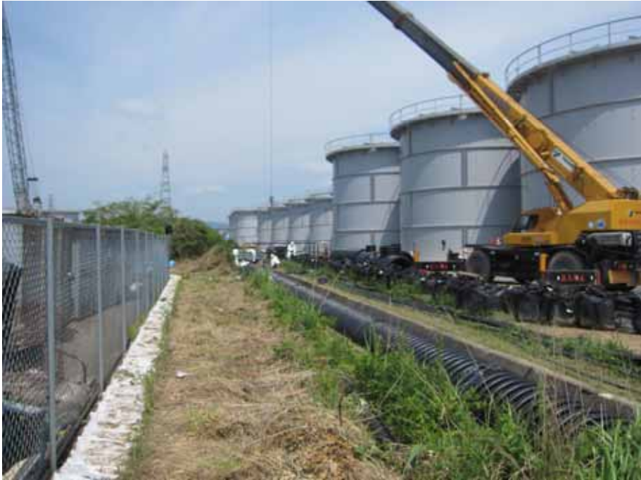
-1 PE pipe installation condition Photo taken by a TEPCO employee on June 18, 2012
