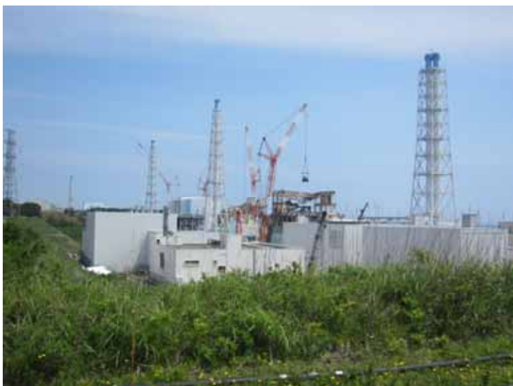
-1 Appearance of Unit 2-4 (View from the southern hill) Photo taken by a TEPCO employee on June 18, 2012
