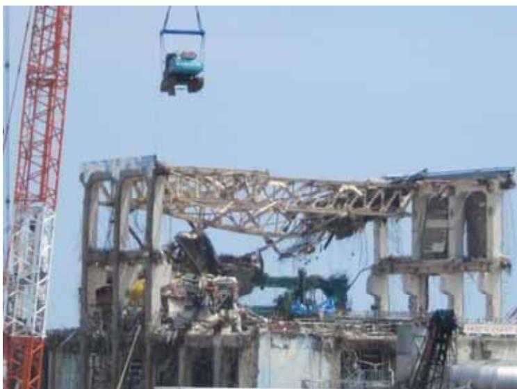
-3 Appearance of Unit 4 (View from the southern hill): Lifting heavy machinery down from the operation floor Photo taken by a TEPCO employee on June 18, 2012
