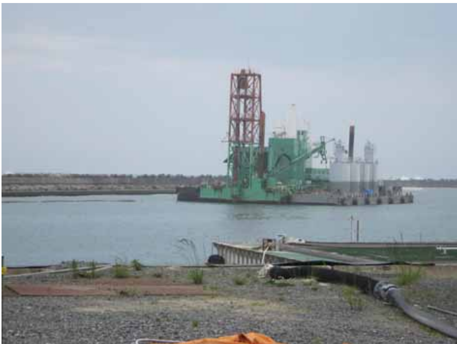
-1 Marine soil covering work: Solidification agent mixer ship (Left), Silo ship (Right) Photo taken by a TEPCO employee on June 7, 2012
