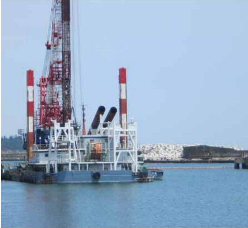
Impermeable wall piling ship Photo taken by a TEPCO employee on June 18, 2012
