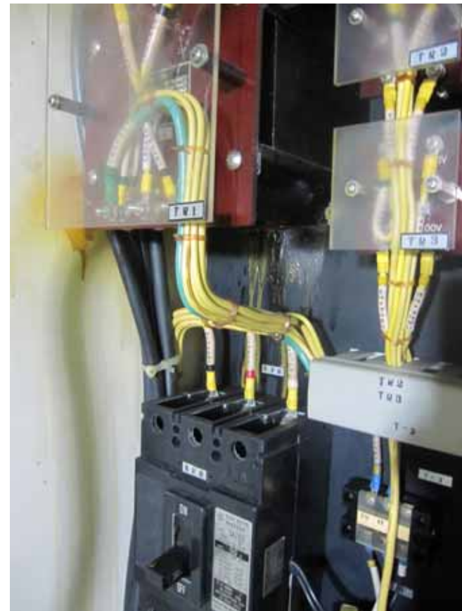
Location where smoke was coming out from (Inside the control panel)
