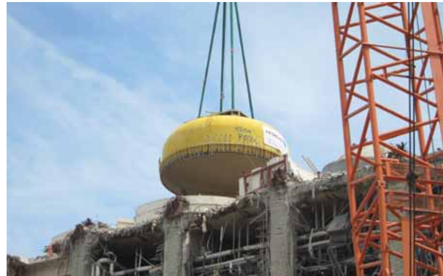
PCV upper lid being lifted up in the upper part of the operating floor
