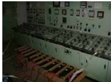
Temporary Batteries were used to supply power to instrumentation
