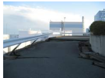
Sagged Road in the Site
