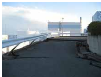
Sagging of Road
