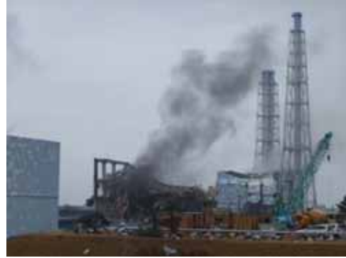
External View of Unit 3 after explosion
