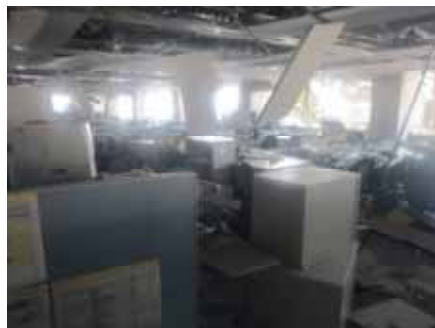
Main Office Damage
