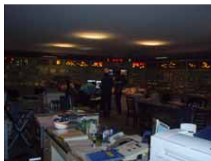
Unit 5/6 main control room: Unit 5 side (Lighting only from emergency lights)
