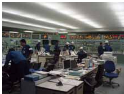
Unit 5/6 main control room: Unit 6 side
