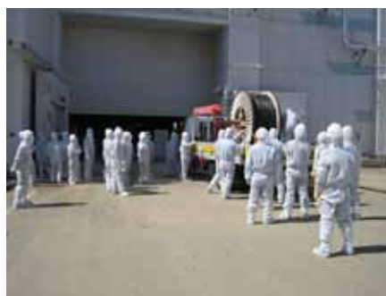
Preparations for laying temporary cable (photo of work conditions at a later date)
