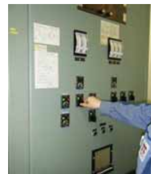
Valve operation at main control room AM panel (photo of work conditions at a later date)
