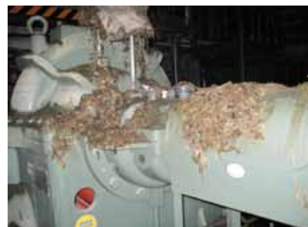
Seawater pump that had been deluged with water (photo taken at a later date)
