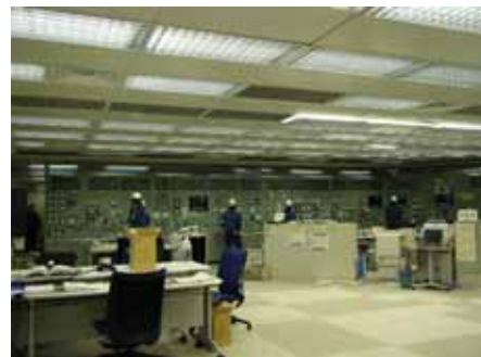
Main control room immediately after tsunami
