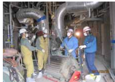
Pump motor recovery work (photo of work conditions at a later date)
