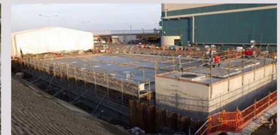
Foundation work being done next to the Unit 7 turbine building (picture taken following concrete pouring)
