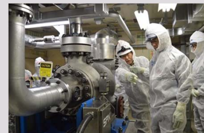
The Mayor of Kashiwazaki City observes the installation of Unit 7 high pressure substitute coolant injection pump
