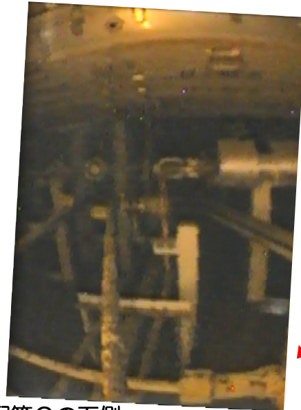
主蒸気配管Cの下側
