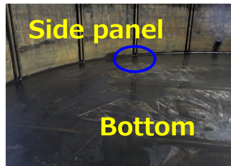
【Reference】 Photo from inside a tank of the same type (after being drained)
