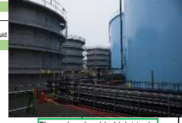
Flanged and welded-joint tanks
