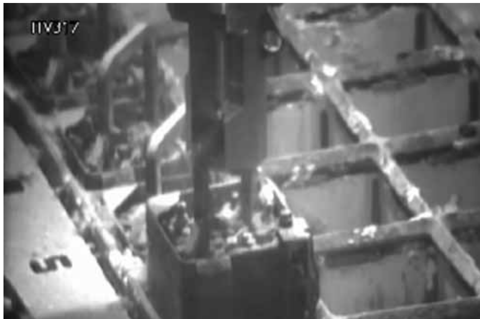
Hoisting the 284 th fuel assembly (Marks removal of over 50% of remaining fuel)
