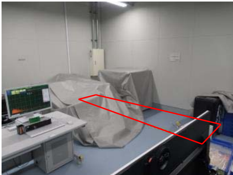
LEPS to be installed here (Inside the chemical analysis building measurement room)
