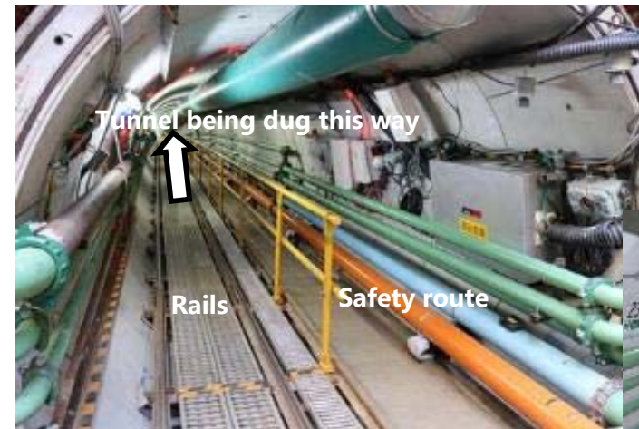
Safety equipment inside the tunnel
