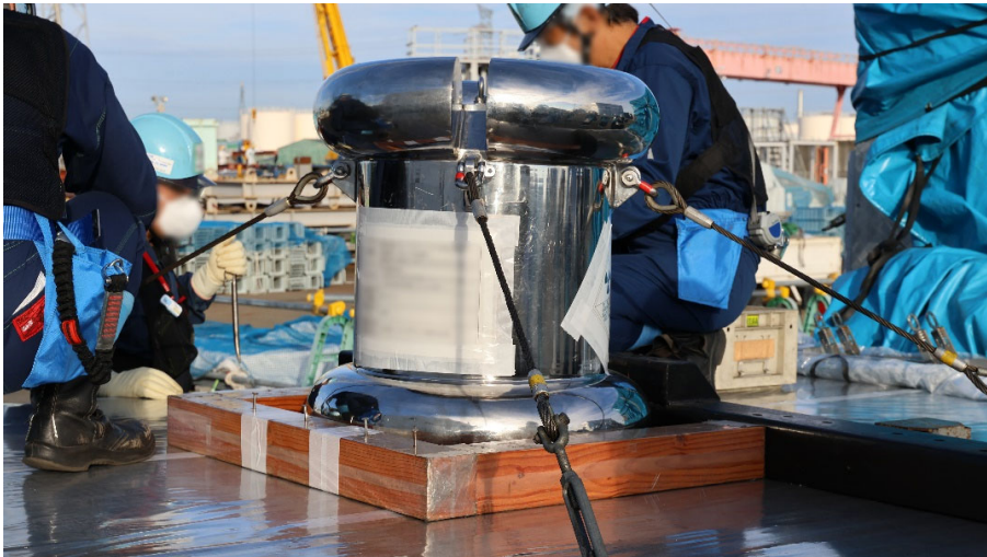
Photo 1: Off-site transportation container loaded onto an off-site transfer vehicle (Photographed on November 12 at 7:50 AM)
