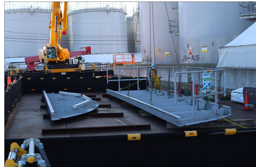
<The top lid removed from J9 area tank> (Photographed at 8:50 AM on February 14)
