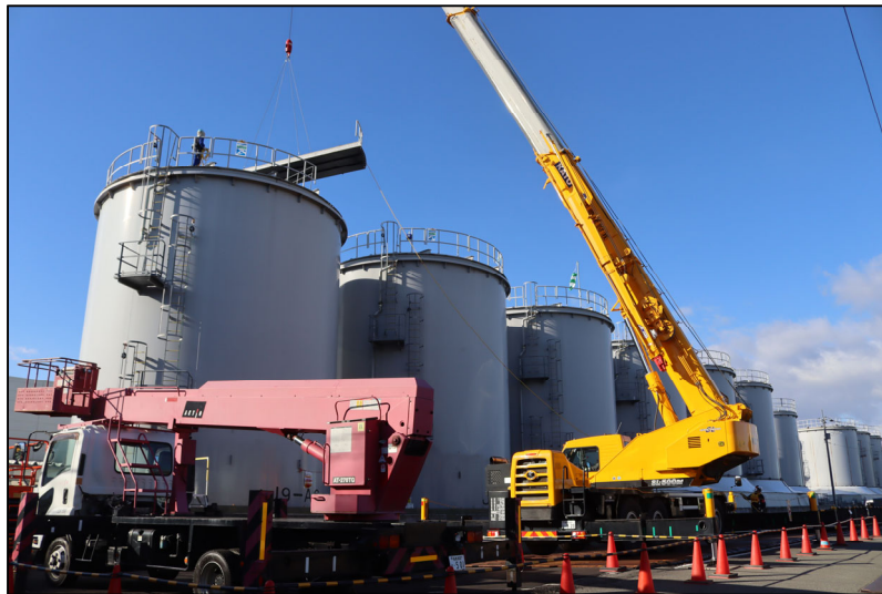
<Removing the top lid from J9 area tank> (Photographed at 8:47AM on February 14)
