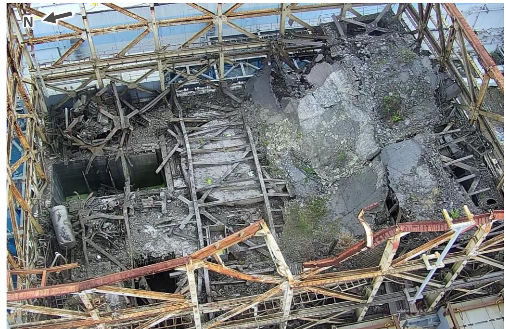
Rubble conditions (prior to large cover installation)
