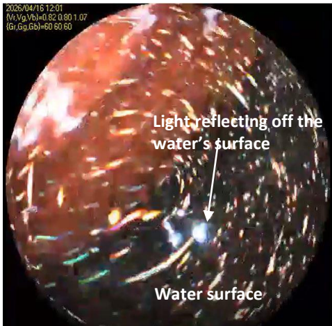
Photo ⑦ Approx. 5.5m below the N16A nozzle
