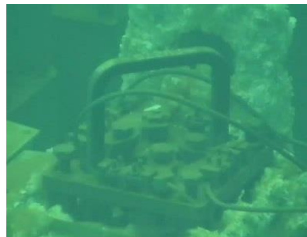
Photograph of the top of the fuel assembly that has been repaired with a wire (Photographed on July 8, 2026)
