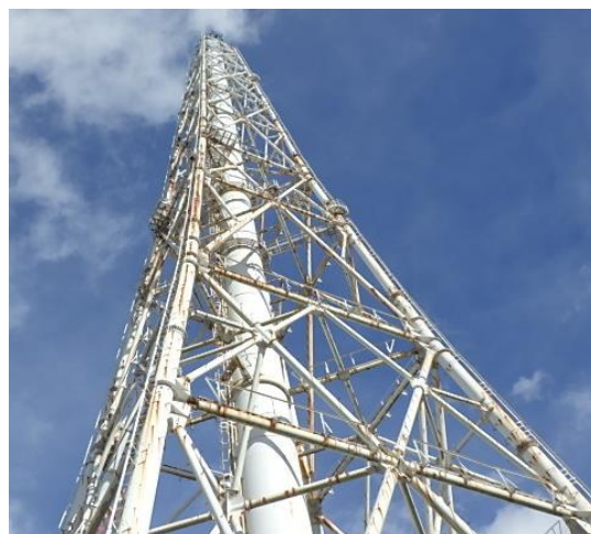
Exhaust stack (photographed on January 23, 2026)
