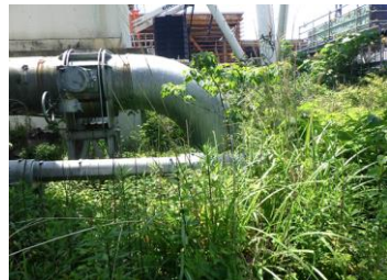
Weeds in the vicinity of the exhaust stack
