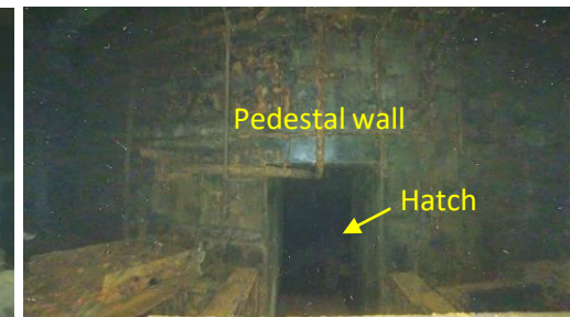
③ : External view of the CRD replacement hatch
