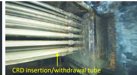
③ : CRD insertion/withdrawal tube (northwest)
