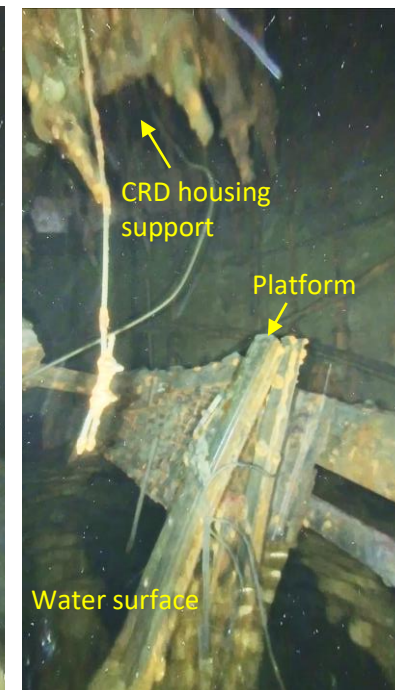
③ : CRD replacement machine ancillary equipment (Platform)
