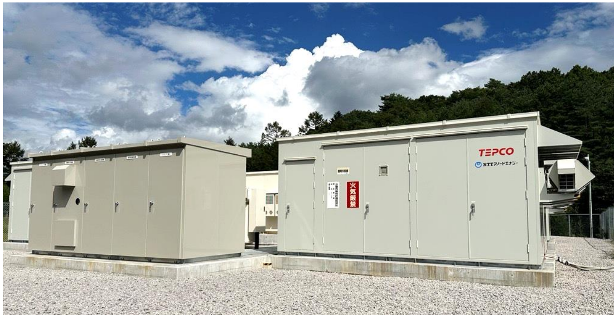
Tsumagoi Battery Storage Station
