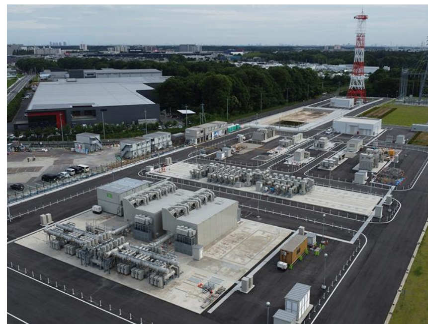
Chiba Inzai Substation
