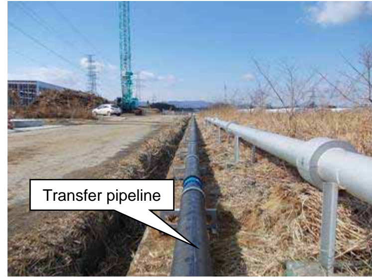
Transfer pipe from A system to the temporary storage tank
