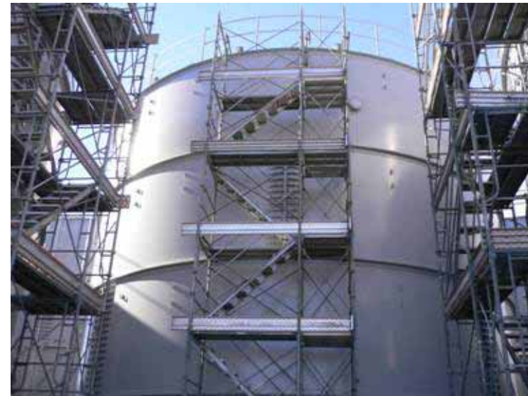
Temporary storage tank
