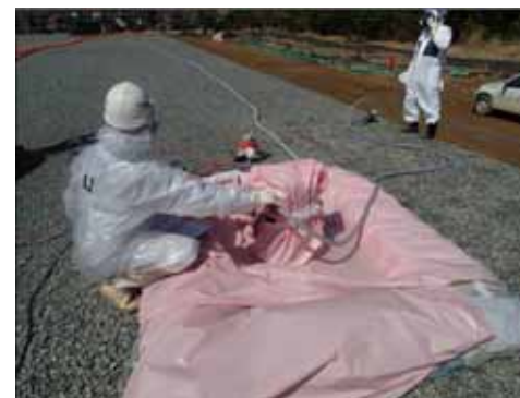
Work to prevent the expansion of contaminated water performed in the northeast side of the leakage detection hole of the underground reservoir No.1
