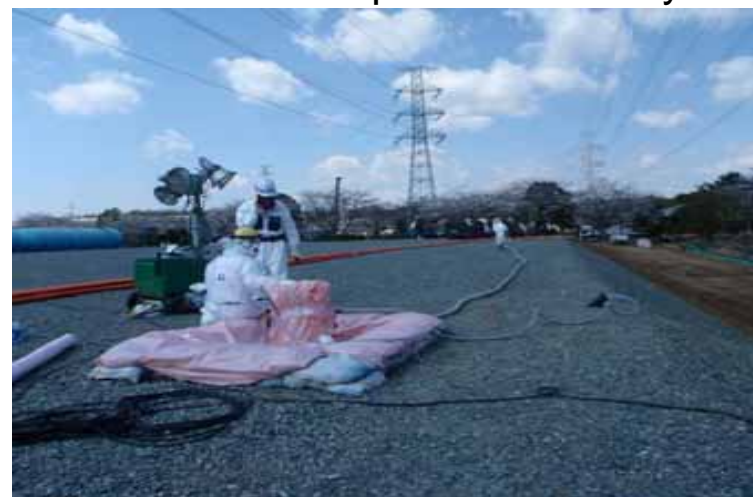
Work to prevent the expansion of contaminated water performed in the northeast side of the leakage detection hole of the underground reservoir No.1
