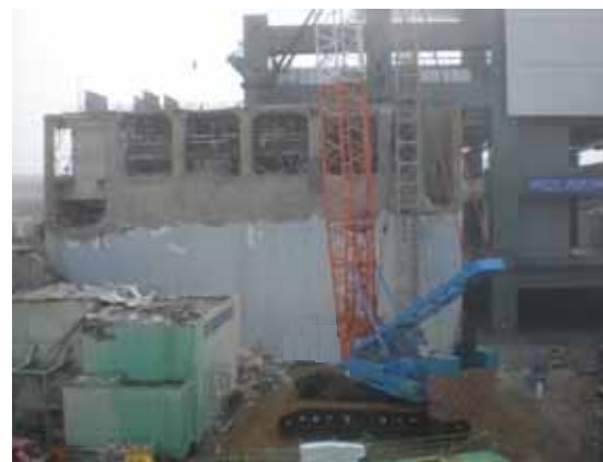
⑤ West wall (Outer surface)
