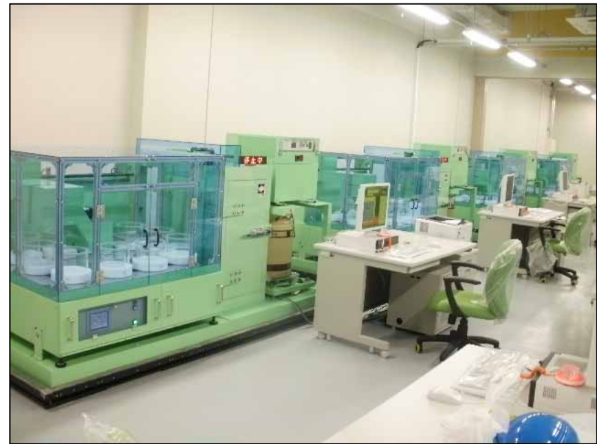
Ge semiconductor detectors installed in the new laboratory (in the first basement)
