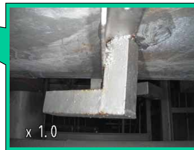
Picture point (5): Clearance in the upper part at the wall surface side (4.3m from the floor)
