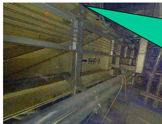
Picture point (5): Upper part at the wall surface side (3.5m from the floor)
