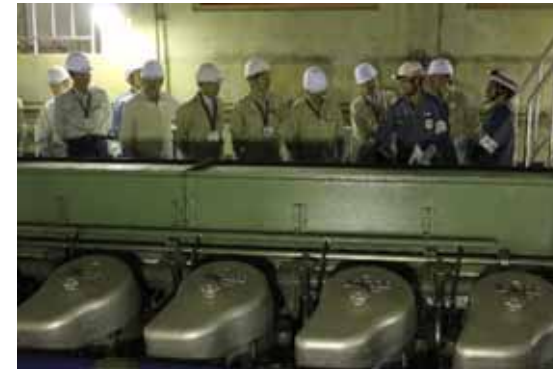
Emergency diesel generator (diesel engine) (in the 2 nd basement of the Reactor Building Annex)
