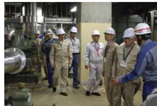
Residual Heat Removal equipment cooling system pump (on the 1 st floor of the Seawater Heat Exchanger Building)
