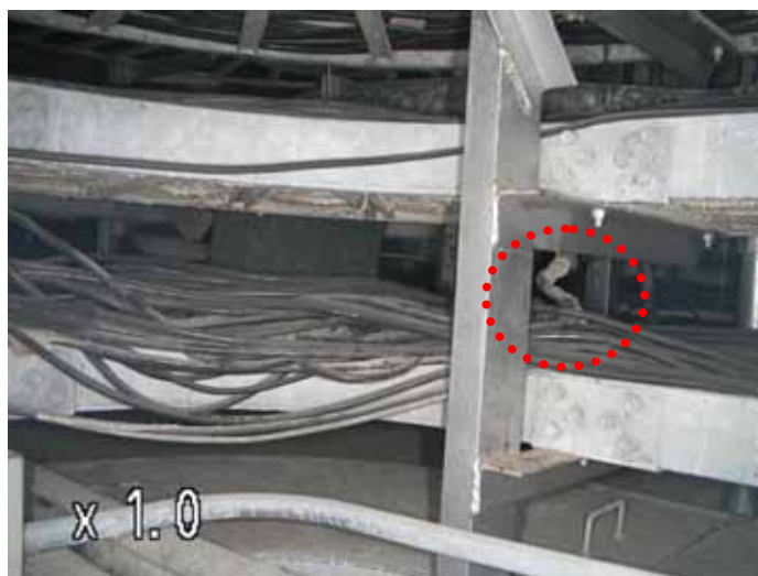
(4) Picture point [2] Upper part of the personal airlock room (5.2m above the floor)
