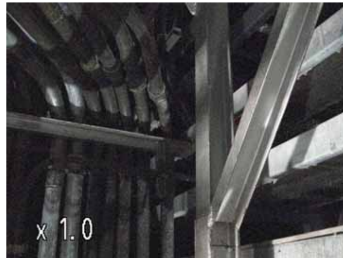
(1) Picture point [1] Upper part of the personal airlock room (4.4m above the floor)
