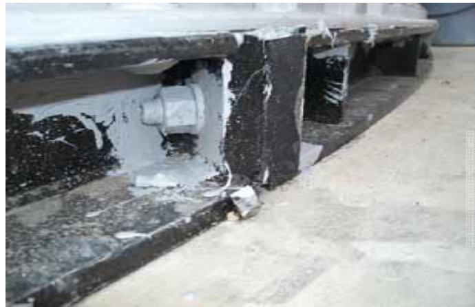
Photo of the joint part of flange at the bottom of the tank
