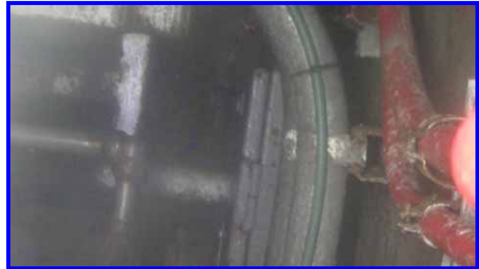
Around OP.7,200: We could not check due to the interference with obstacle
