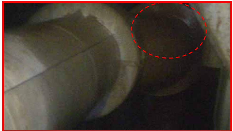
Around OP.5,900: We found that water was dropping from the upper part
