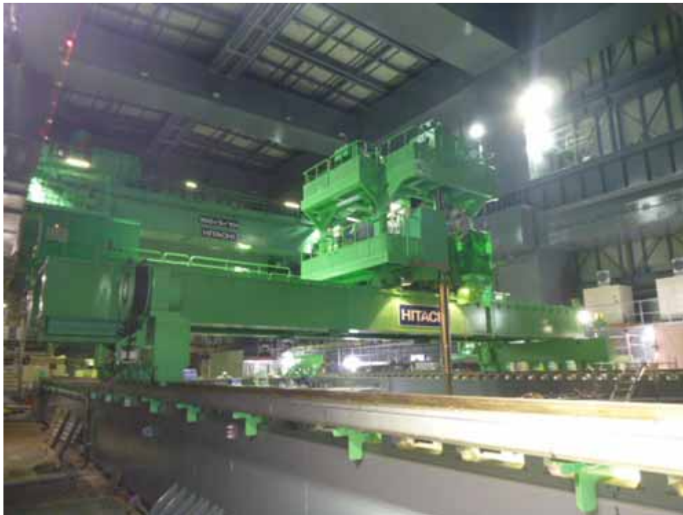
Source: Photo taken by TEPCO on September 19, 2013
