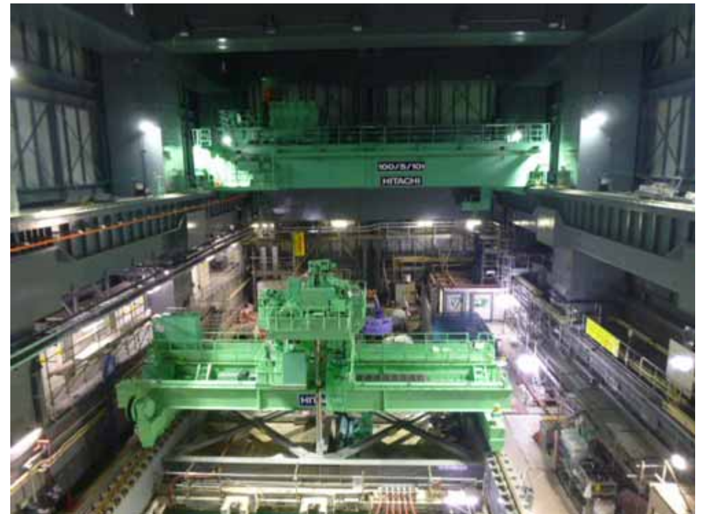
Source: Photo taken by TEPCO on September 19, 2013
