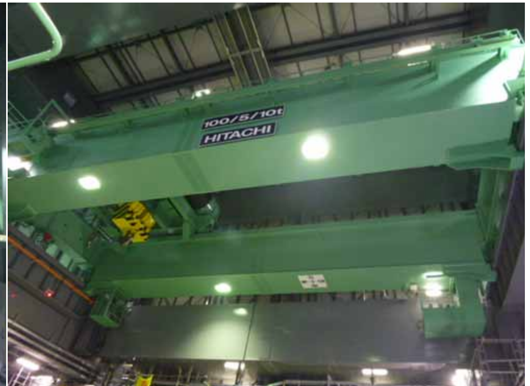
Source: Photo taken by TEPCO on September 19, 2013
