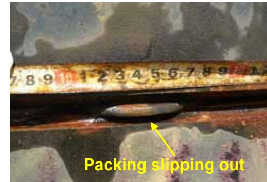
Leak path part on the backside the bottom plate before removal
