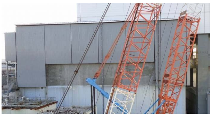
⑤ West wall (outer surface)
