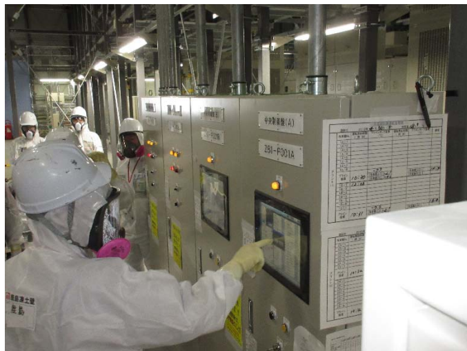
Starting up refrigerators
