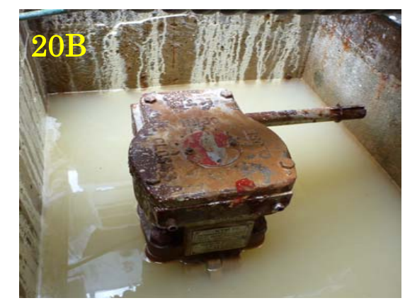
Fuel Pool Cooling and Filtering System Valve
