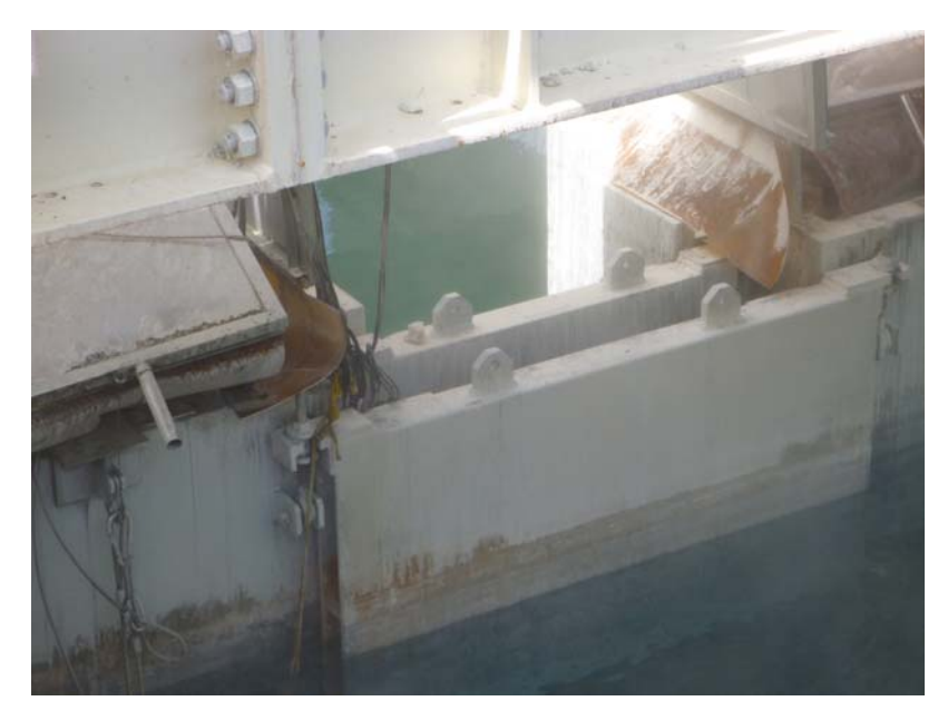
Spent Fuel Pool Gate
