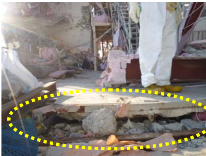
③ Floor pushed up
