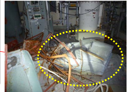
⑰ Rubbles from air-conditioning ducts
