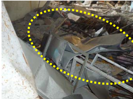
⑬ Damages to the floor
