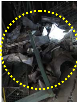
⑮ Rubbles from air-conditioning ducts
