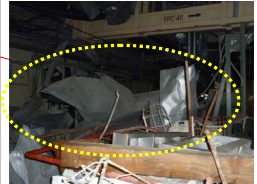
⑯ Rubbles from air-conditioning ducts
