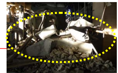
⑩ Rubbles from air-conditioning ducts
