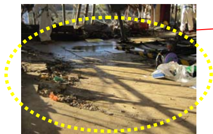
⑧ Floor pushed down
