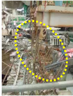
① Rebar deformed upward
