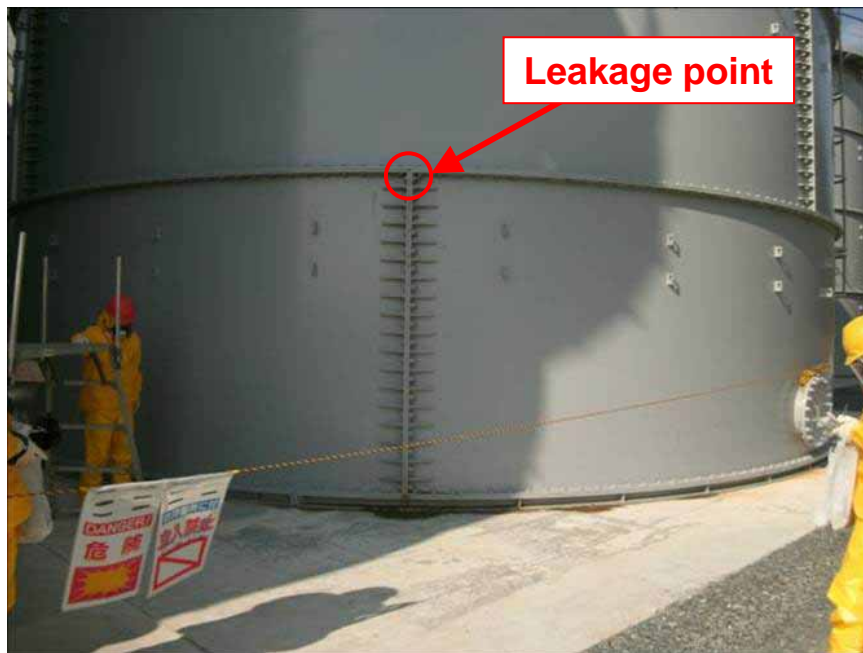
< The tank at which leakage was confirmed >
