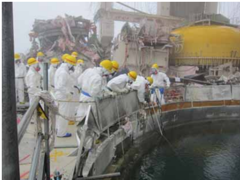
Confirmation of the reactor well on the fifth floor of Nuclear Reactor Building Unit 4
