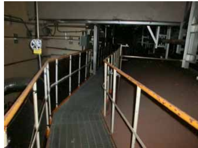
Unit 3 torus room catwalk
