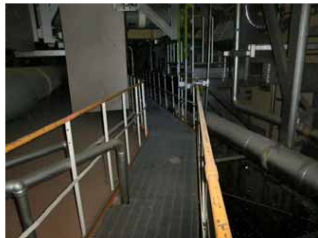
Unit 3 torus room catwalk
