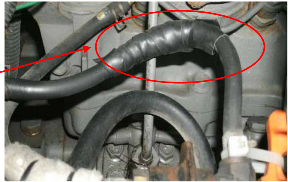
After emergency measure implementation (leakage stopped after wrapping tape around the hose)
