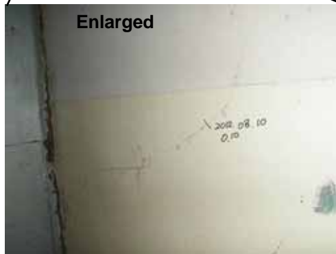
1. Inner surface of the second floor west exterior wall between W2 and W3 (Crack width: 0.1mm)
