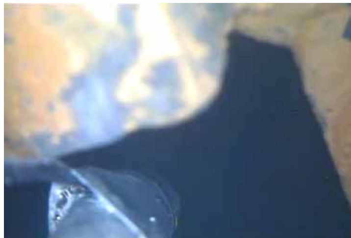
3. Accumulated water (Under water) Photos taken on October 10, 2012 by TEPCO
